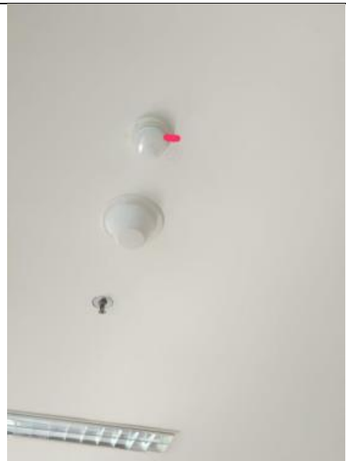
The Automatic Fire Alarm Sensor System
